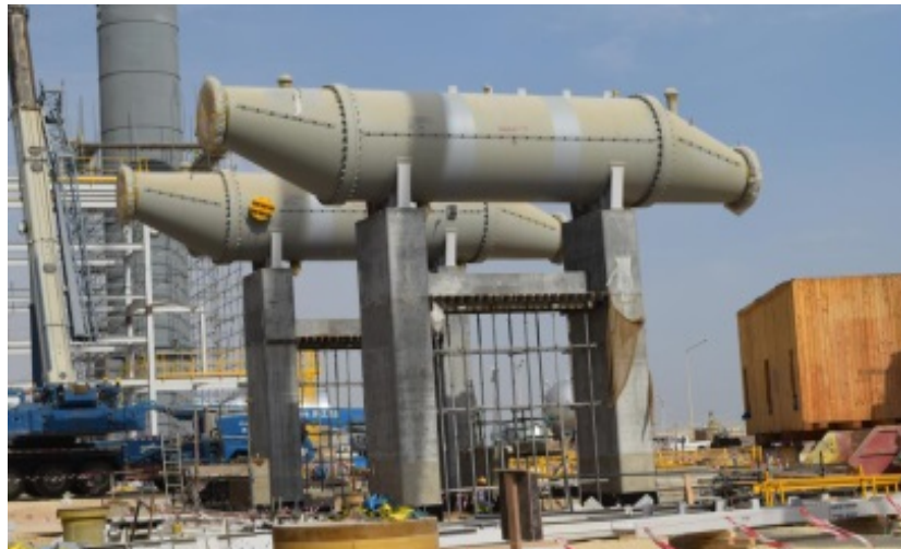
Ammonia Heat Exchangers
