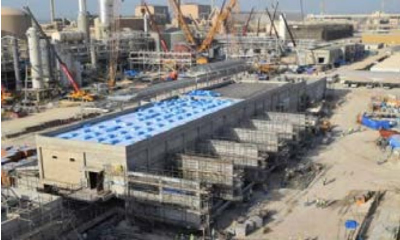
Main Substation / Ammonia Plant
